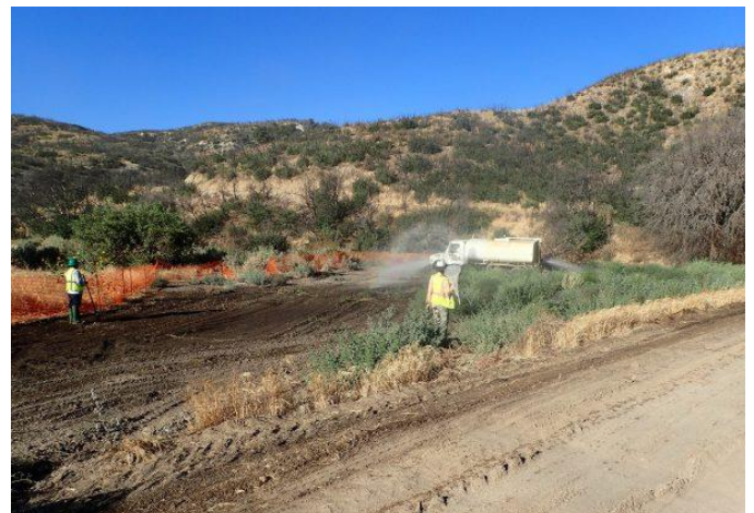
A WRA biologist monitors excavation and dust abatement in one of the restoration areas.
