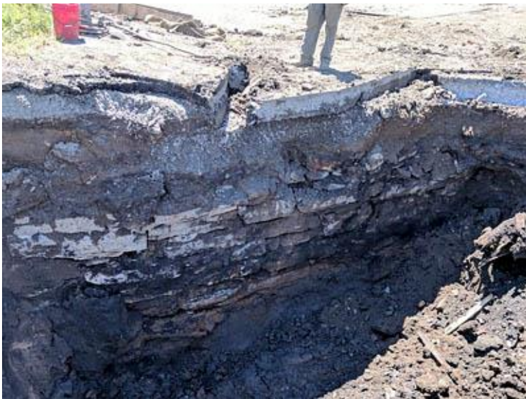
Left: Work stops when a partial wall is exposed along a section of Erie Canal dating from the mid-1800's.
